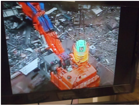
Fig. 14. Remote fuel supply system.
