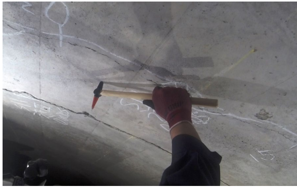
Fig. 1 Hammering test conducted by a professional on the ceiling portion of a tunnel: only a simple hammer is needed thus the popularity of this non-destructive testing method. Still, there is the need of skilled operators to correctly differentiate hammering sounds and given the great population of structures in need of testing, automation is actively demanded. Also, since it relies heavily on the operator's skills, the final result remains subjective
