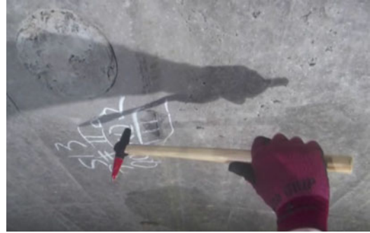
Fig. 1. Hammering test conducted by a professional: a hammer is used to hit the surface of the concrete structure and the returned sound used to assess whether a defect lies beneath the surface or not.
