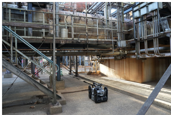
Fig. 1. An inspection robot in a petroleum refinery (ENEOS Corporation).
